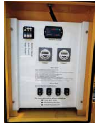
Timer & Switch Panel w/ Battery Fuel Gauge
